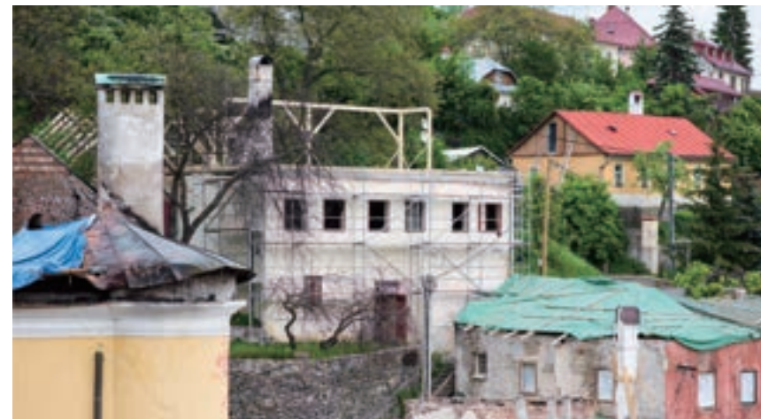
Improvised covering of the damaged houses
